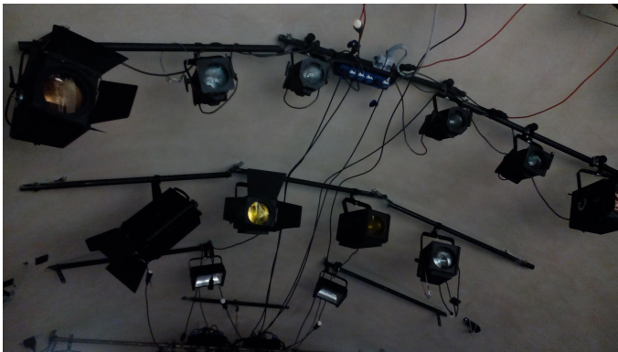
Lighting rig (auditorium)
